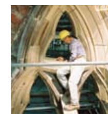
Window treatment: No more drafts! Librarians rejoiced as the 147 leaky leaded windows were restored
